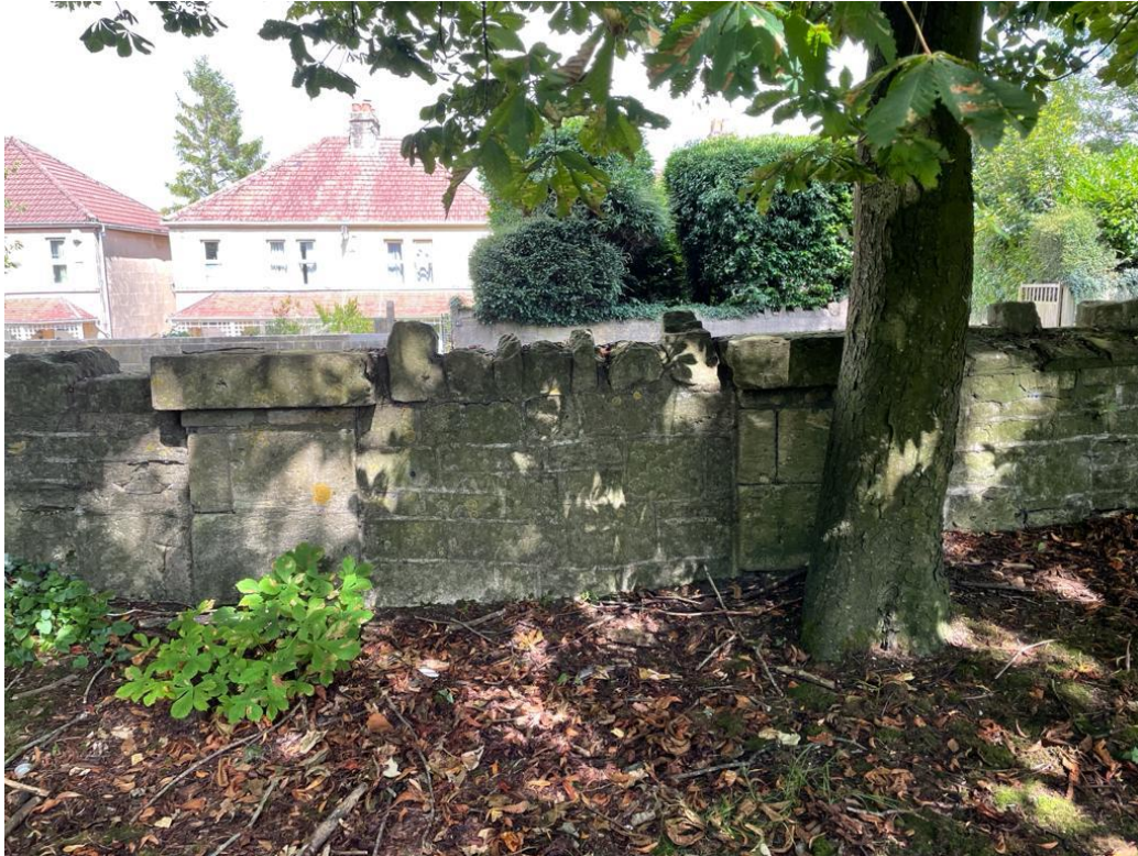
Figure 1: Clear evidence of former gated entrance to the St Martin's burial ground between two brick piers close to Frome House.
