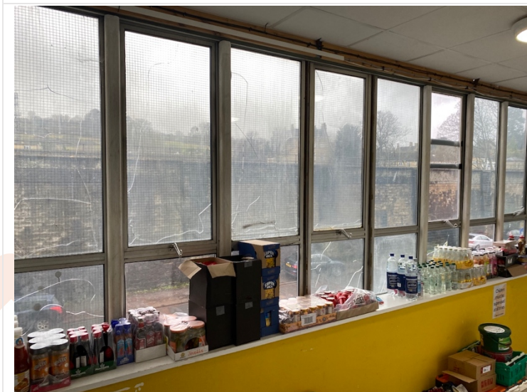
Defective glazing system
