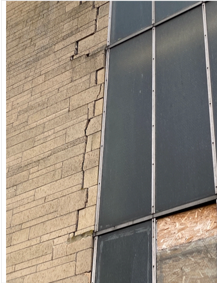
Structural movement to façade
