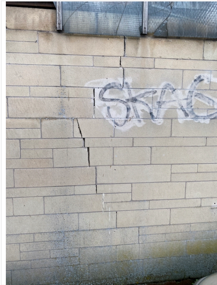
Structural movement to façade
