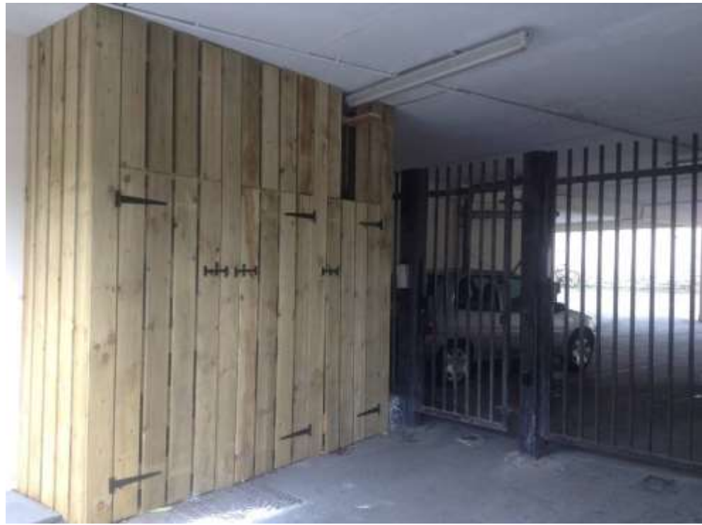
Figure 10. External storage does not exist as shown on plan. Instead there appears to have been a make-shift shed erected at the entrance to the parking providing little and inadequately secure storage for tenants.
