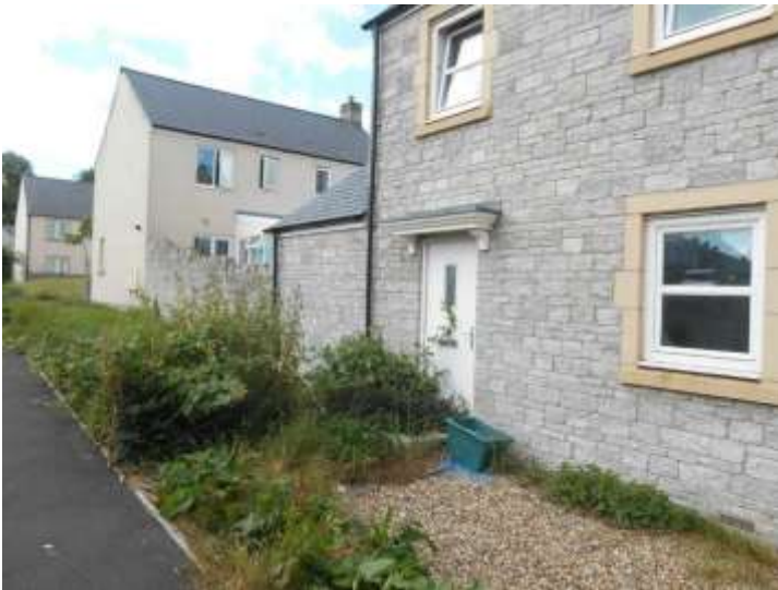
Figure 10 - Overgrown front garden suggesting back door is used as primary entrance to property.
