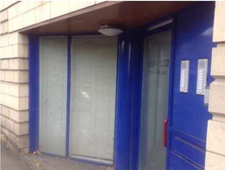
Figure 6. Poorly designed threshold with front door and bedroom window set directly side by side, creating issues of privacy and security.
