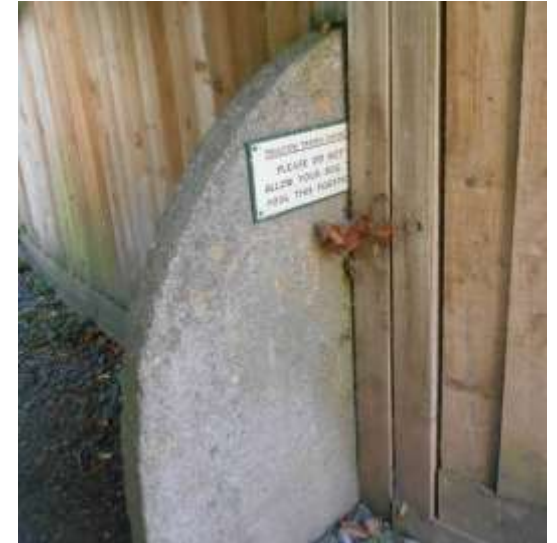
Figure 9 -- Plaque on existing stone work with text covered by poorly placed fencing.
