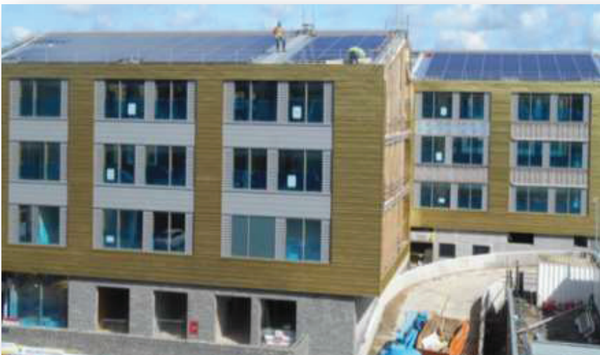
THE 243KWP SOLAR ARRAY BEIGN INSTALLED IN 2014 ON THE COUNCIL'S KEYNSHAM CIVIC CENTRE. THE ARRAY WILL BRING A FINANCIAL BENEFIT OF AROUND £50,000 AND SAVES 125 TONNES OF CO2 PER YEAR
