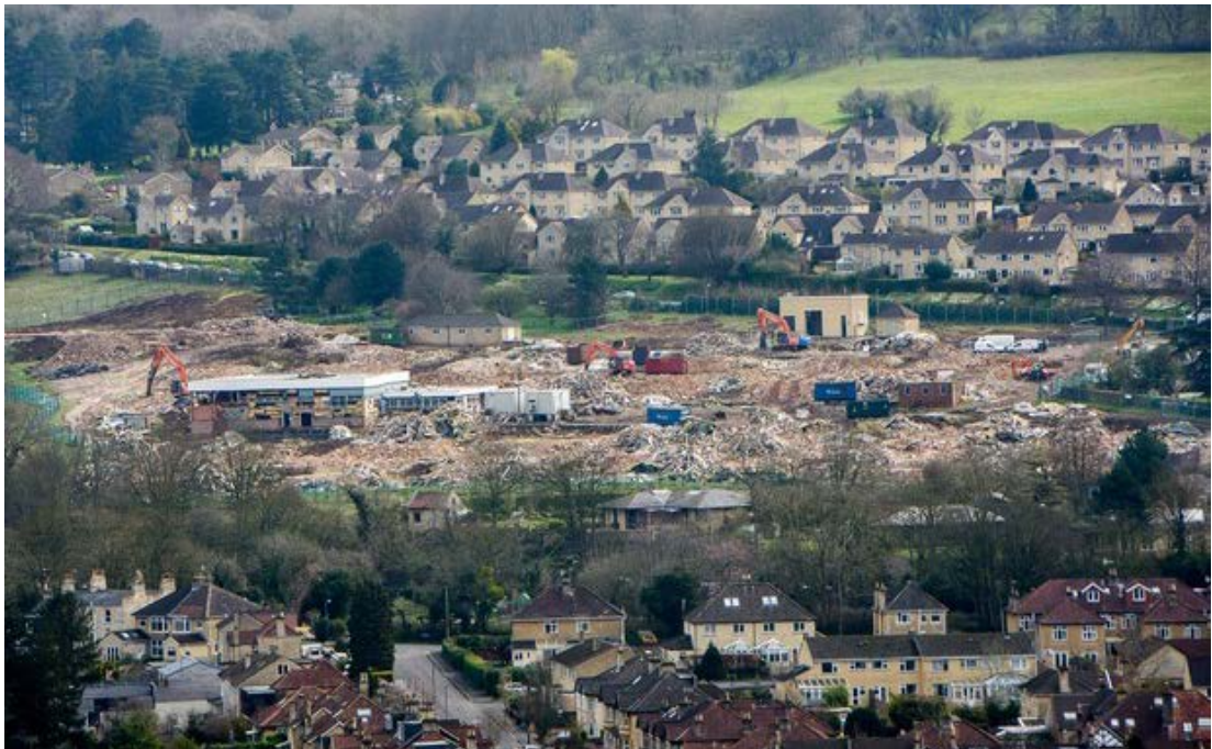
Warminster Road April, 2016. Since purchasing the site Firestone have moved swiftly to demolish and clearance
