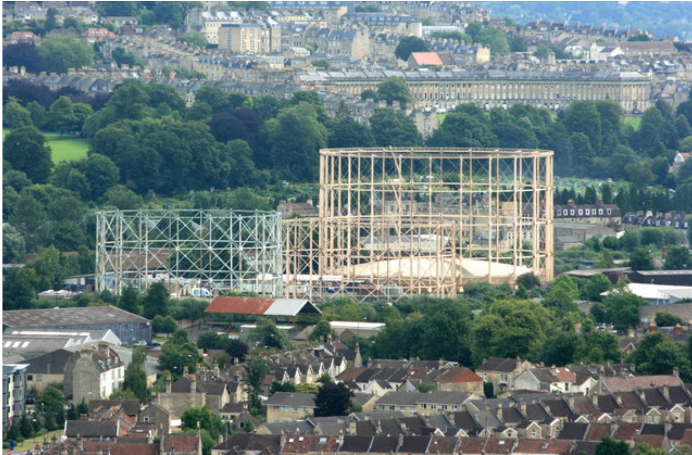
Figure 7: Windsor House Gas Holder Station (note only one gas holder now remains)
