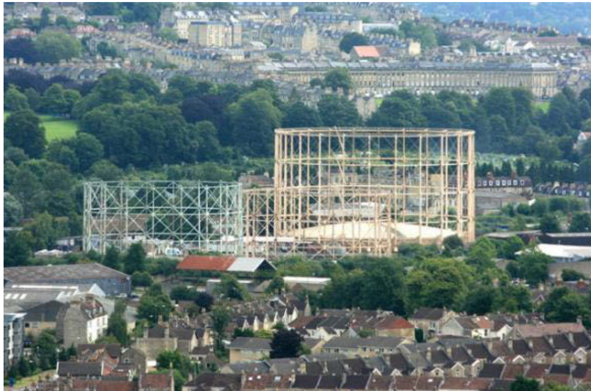
Figure 7: Windsor House Gas Holder Station (note only one gas holder now remains)
