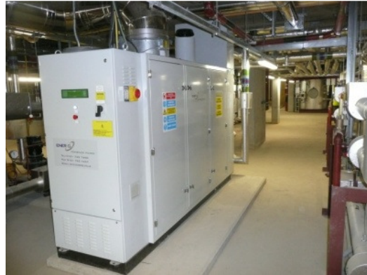
Figure 4 Energ100kWth, 70kW e gas-fired CHP plant, installed at Highbury Stadium redevelopment, London.
