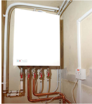
Figure 1: A heat exchanger inside one of the flats connected to the Aberdeen district heating network (Source: Aberdeen City Council: a case study of community heating CE65, Energy Saving Trust, 2003)
