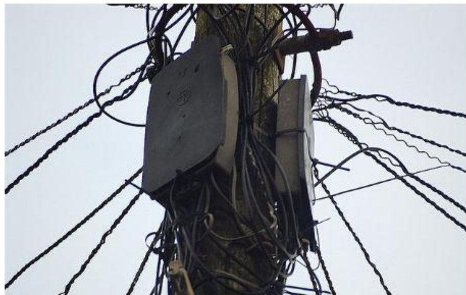
Aging BT Openreach infrastructure
