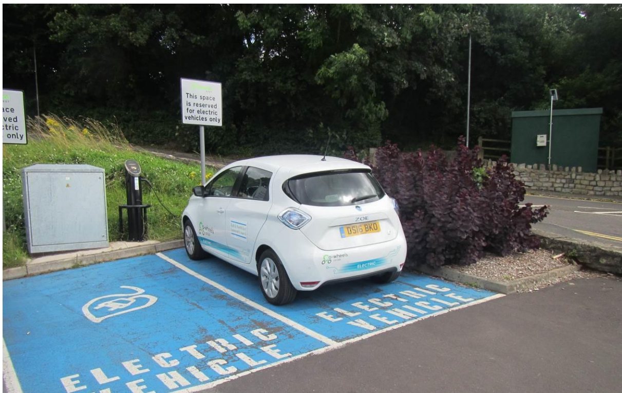
'Source West' electric vehicle charging point in Keynsham.
