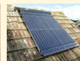
solar thermal panels for hot water
