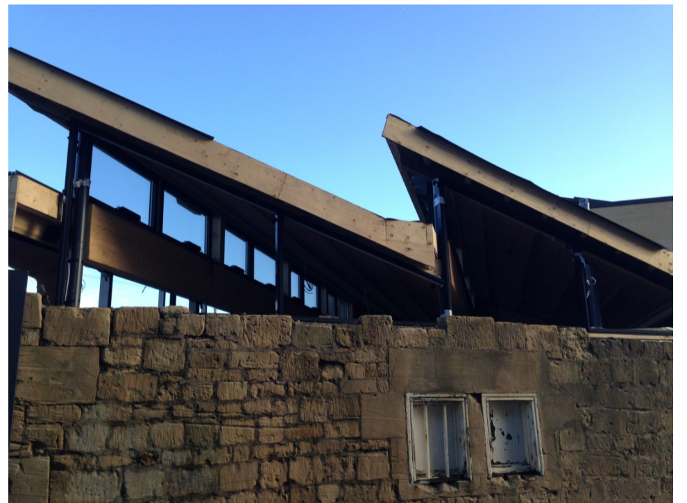
Image 3: Section of photovoltaic panels and preserved existing wall, Rock Hall Lane. Jan 2014.
