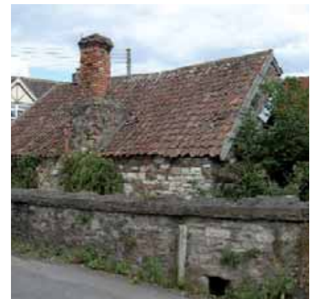
Restoring derelict buildings would enhance the area's appearance
