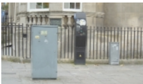
Utility plant and junction box
