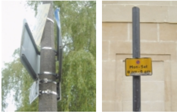
Poorly detailed fixings for signs Pole projecting above sign
