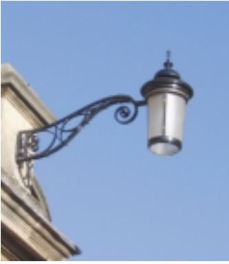
Street lights mounted on buildings
