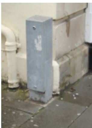
Feeder pillar should be painted black or appropriate colour
