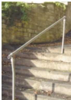
Poor quality railings
