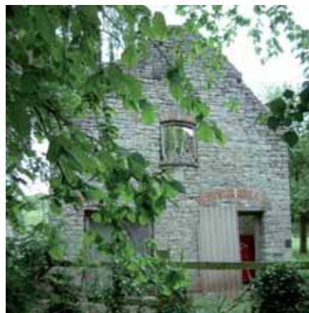
The ruins of the Tannery would benefit from continued maintenance
