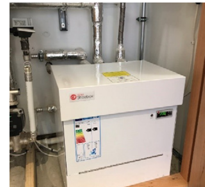
Ground source heat pump
