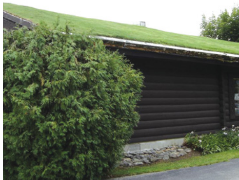
Green roofs can help reduce pollution and surface water run-off and are particularly useful in dense urban areas.
