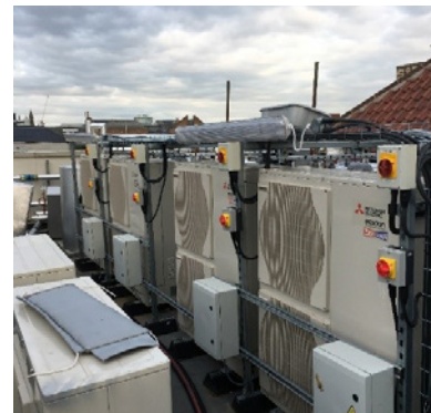
Air source heat pump
