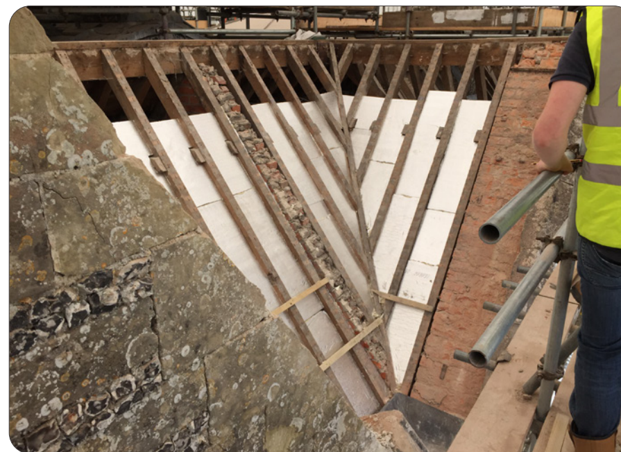
Each eaves detail needs careful thought once insulation is added. Often bespoke solutions have to be devised to achieve effective improvement
