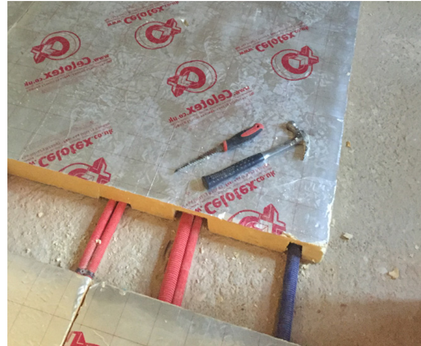
Photo showing insulation with integrated underfloor heating retrofitted to an existing solid floor.
