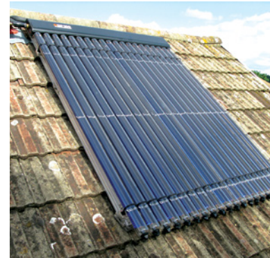
Solar thermal panels for hot water
