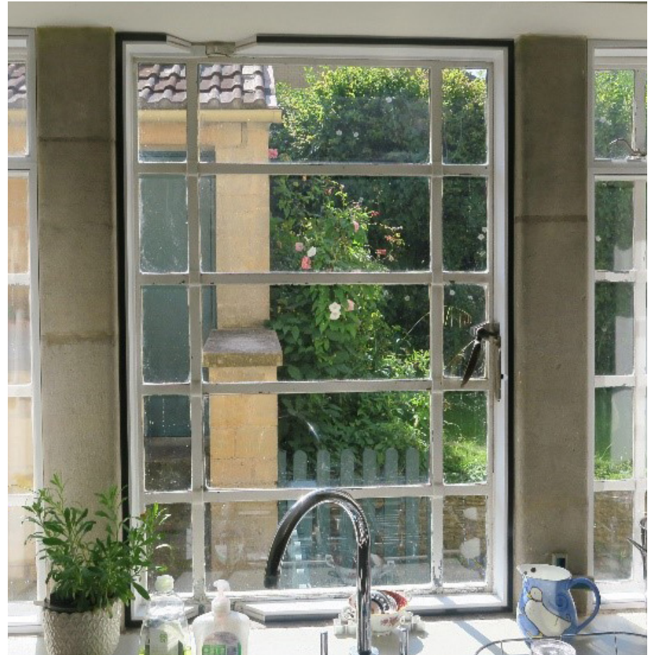
Secondary glazing in metal framed windows, St Alpheges Presbytery, Bath. Photo copyright: Bath Preservation Trust.
