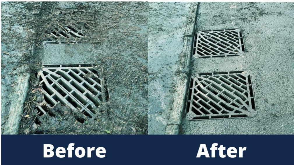
Mud and leaves cleared from gutters in Southstoke in Combe Down
