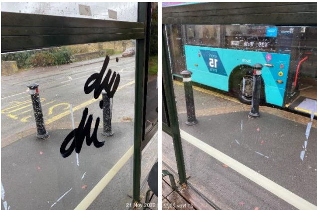
Graffiti removed from a bus stop on Newbridge Road, Newbridge
