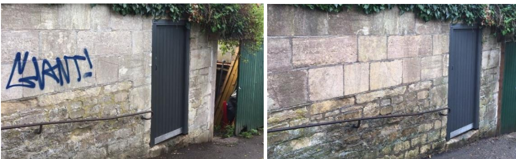
Graffiti removed from a domestic property on Sydney Buildings in Bath
