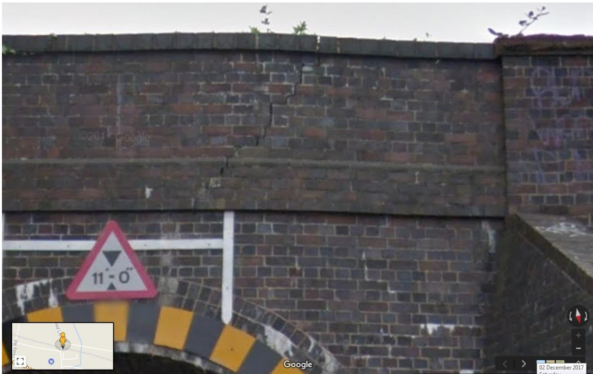
Figure 3.3: Broadmead Lane Bridge - Cracking in the south parapet and distortion of the horizontal alignment indicates foundation failure
