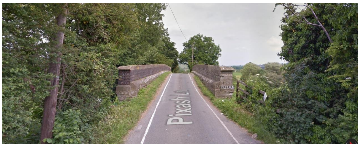
Figure 3.9: Width restriction and blind summit at Pixash Lane Bridge
